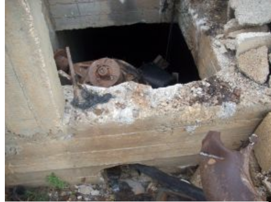
'Umar demolished well, Jenin governorate, October 2012 – Al-Haq©
